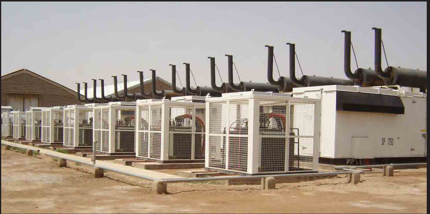
Tameen Southeast generating facility will soon be fully operational and providing 11 megawatts of additional electricity to the Ramadi grid.
