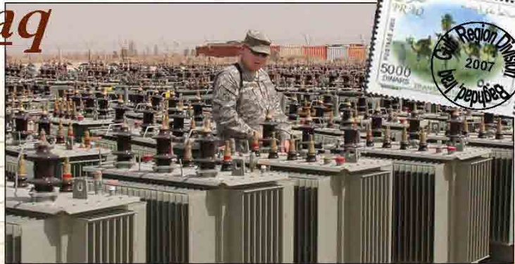
SFC Johnson checks electrical materials for Fallujah
