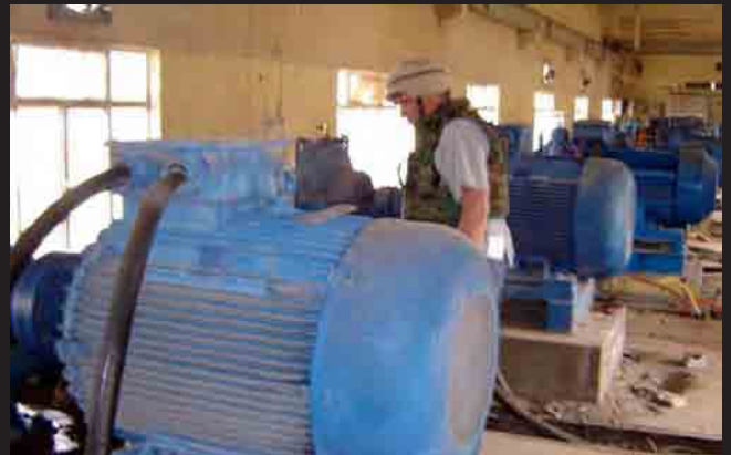
Kabeer Water Treatment Plant in Ramadi is getting new pumps and other extensive repairs.
