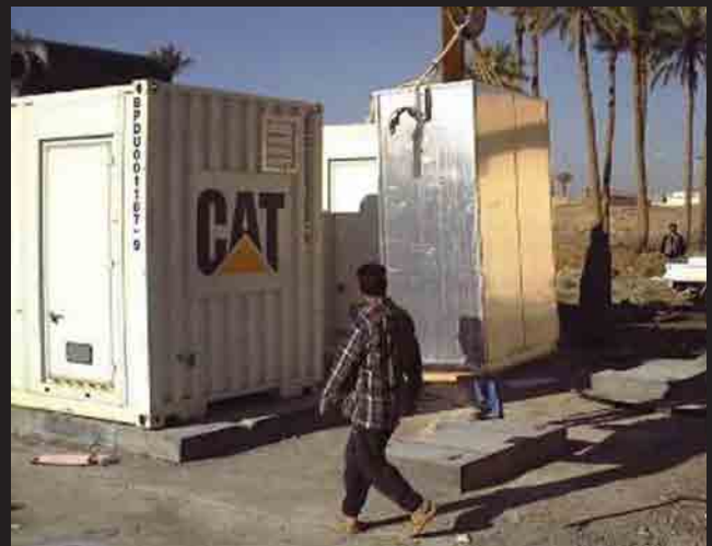
Two new generators at the Kabeer Water Treatment Plant in Ramadi will ensure uninterrupted power for that essential service facility.
