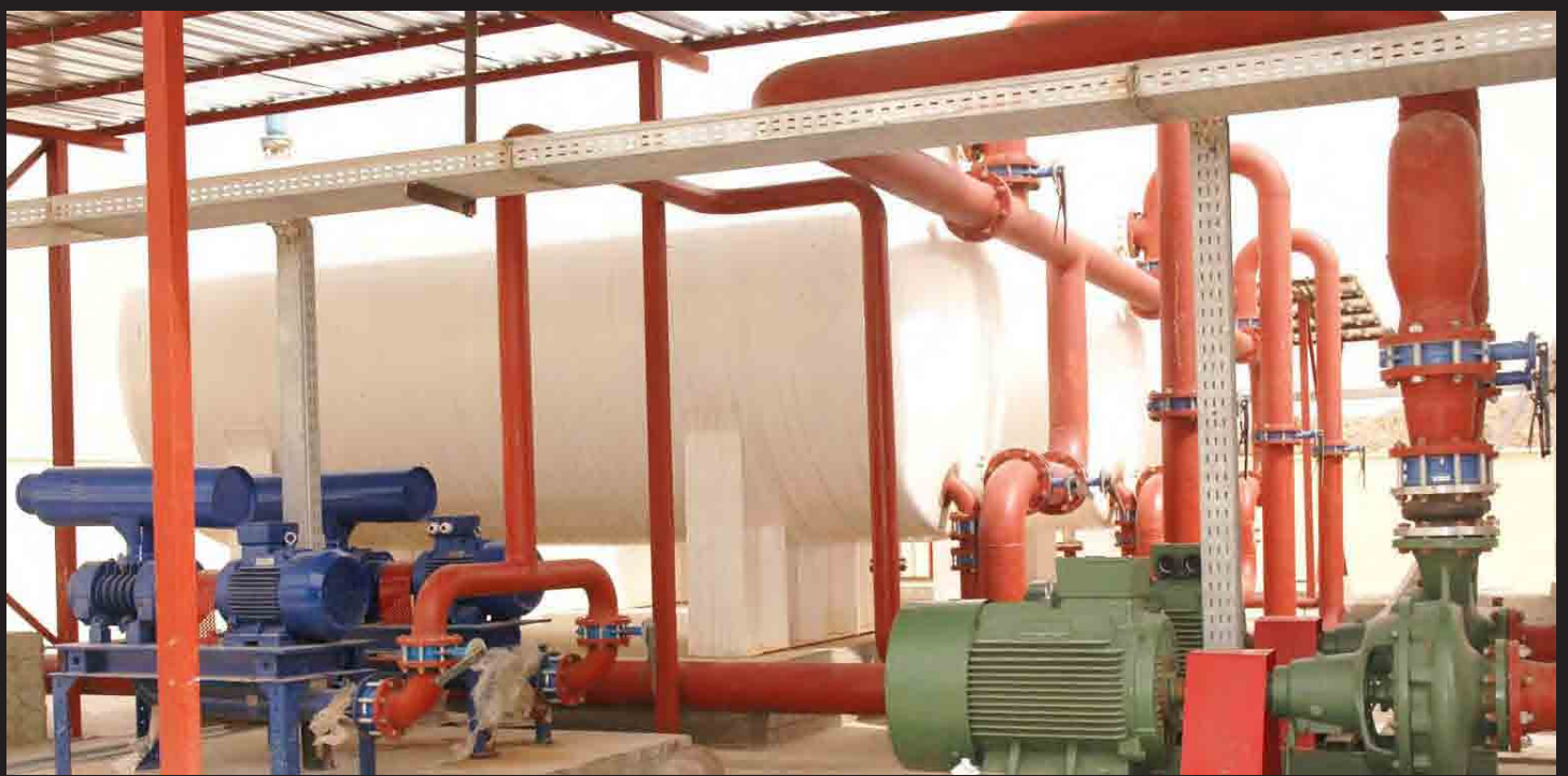
One of the dozens of water compact units being constructed for villages throughout Al Anbar Province.
