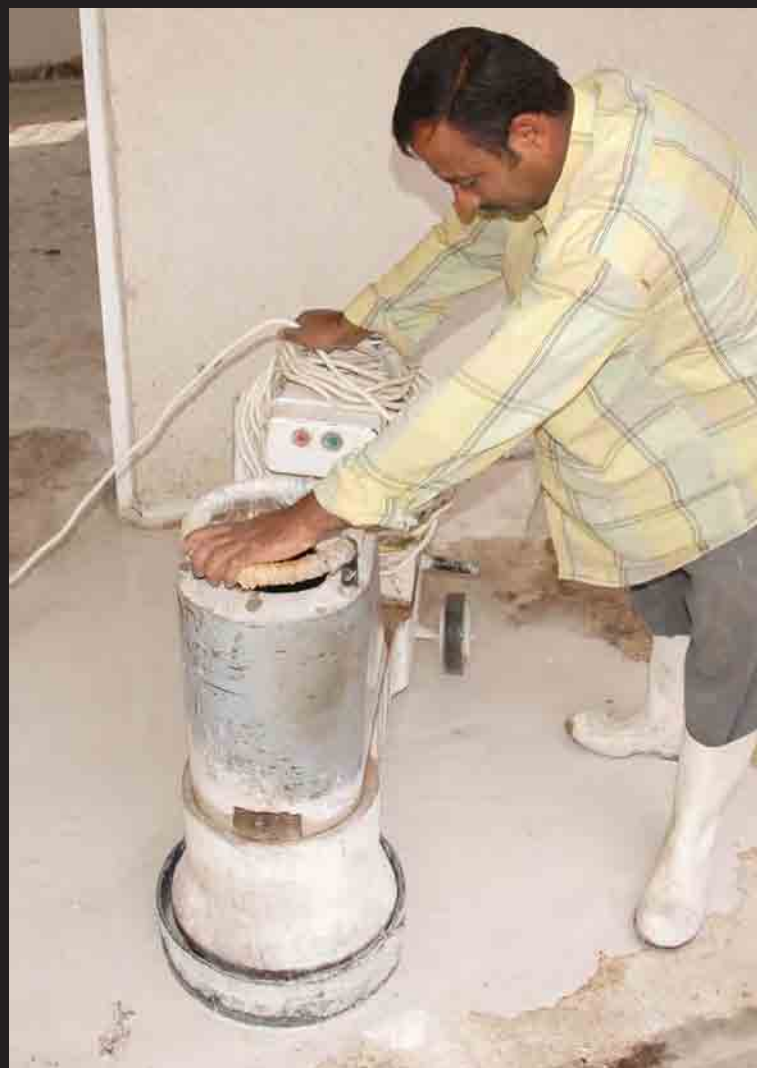
Polishing the new floors along with some electrical and masonry work are among the final items remaining to be finished to open a new primary school in north Baghdad.
