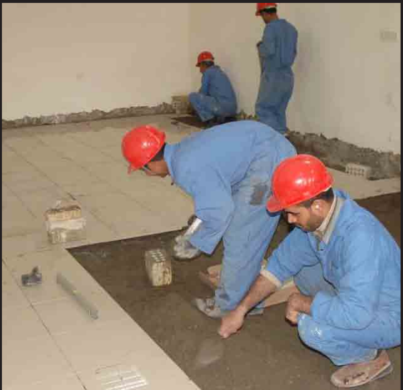
Workers install the floor in the new addition for the Kadamiyah Courthouse complex. Work on the project started in August and should be completed in May. Kadamiyah Courthouse has about 300 litigants attending the court daily.
