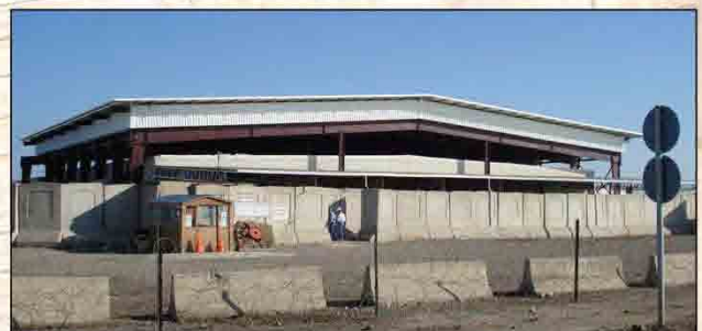
Two of the seven overhead protection projects at Victory Base near the Baghdad International Airport
