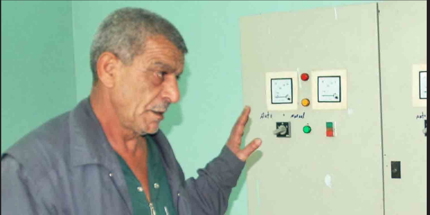
Kadamiyah Sewage Lift Station operator shows two of the new electrical panels at his facility.
