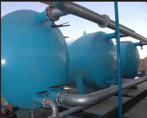
The new Al Askari Water Treatment Plant is currently under construction and when finished will provide water to homes in Fallujah's northeast quadrant.
