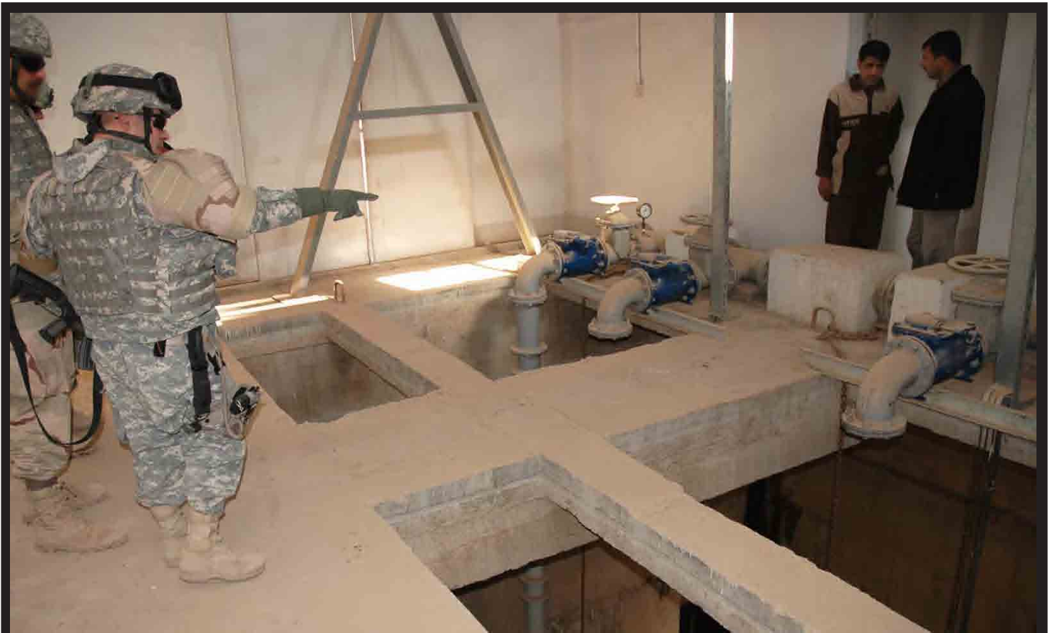
Maj. Robert Nash with the U.S. Army Corps of Engineers checks one of the sewer lift stations being rebuilt.
