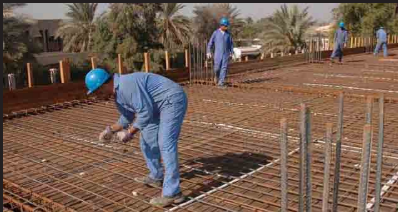
Iraqi workers prepare to place concrete at the Academy of Health and Science in Baghdad
