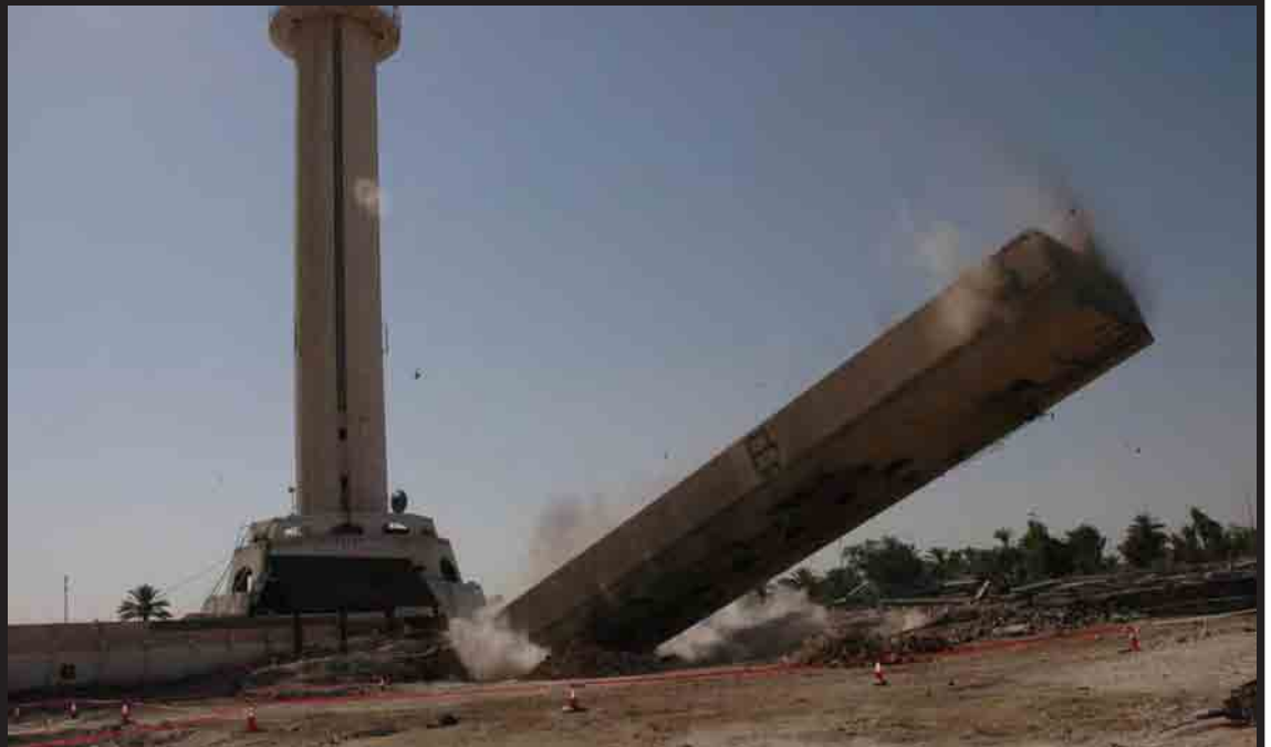
A 13-story concrete stairway is removed Aug. 5, clearing the site for the new $22.7 million Al Mamoon Exchange and Telecommunications Center for Baghdad.
