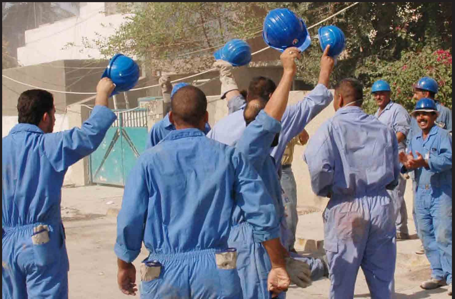
Iraqi workers celebrate after successfully pulling down a 13-story concrete stairwell Aug. 5 as they clear a site for the new $22.7 million Al Mamoon Exchange and Telecommunications Center. In all, 70 Iraqi workers are employed there now and that number will grow to about 400. For Saturday's demolition, Iraqi Army troops blocked off the nearby street to ensure security and safety. "We're doing this for the Iraqi people," the First Sergeant in charge of the detail said. "We're very pleased this new facility is being built."
